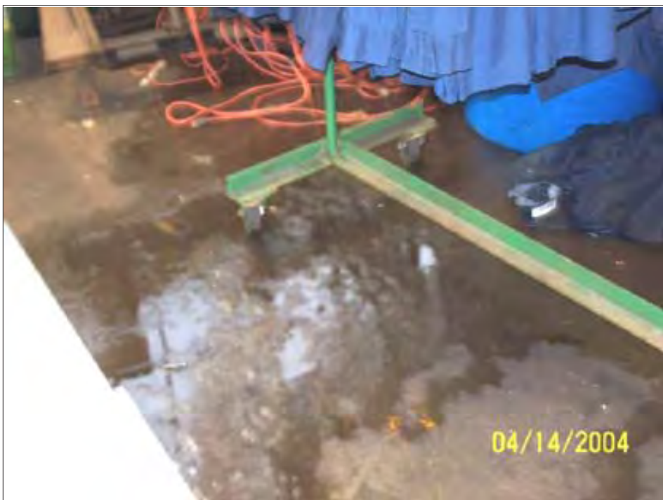
Another aspect of the wet floor at the Municipal Garage as a result of the rain coming through the roof.
