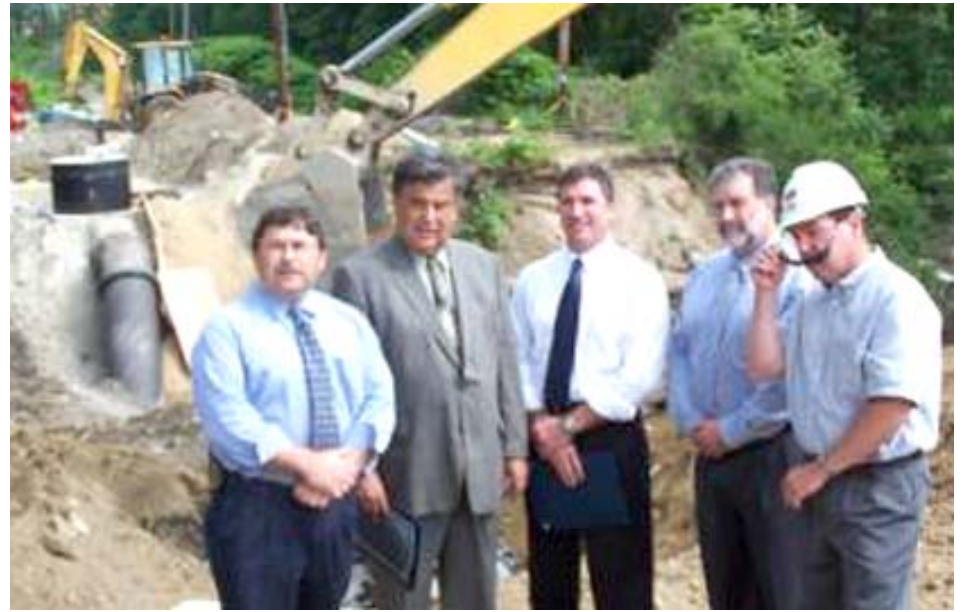
From left to right: Paul Jessel of waste water division, Mayor Fiorentini, Robert Ward waste water division, Fred Haffty for waste water and Joseph Barbone of Methuen Construction which handled the project.
