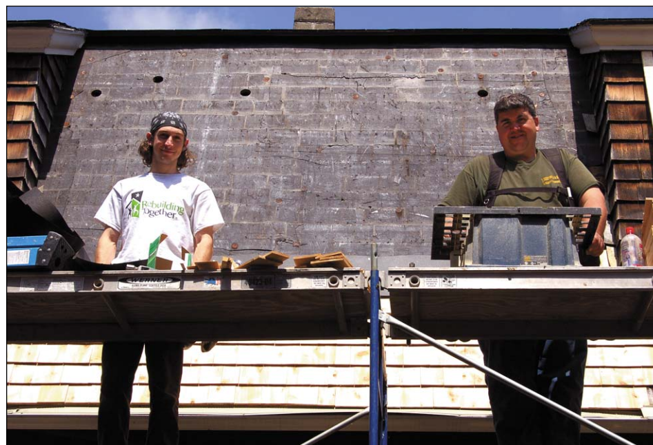
Ryan McCarthy and Jay Martinoli were busy repairing the roof of a house. In Haverhill, over 300 volunteers worked on 37 homes.
