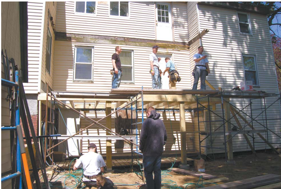
Looking at the porch from left are R. J. Mailloux (Mailloux Brothers Construction Company in Methuen), Jake Morton, David Dubois, Joe Sherlock, Russ Mailloux and Keith Webb. The replacement of this two-story back porch and stairs would have cost over $30,000 to the homeowner.
