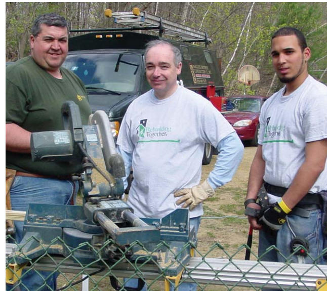
Some volunteers replacing two doors, building a back porch and refurbishing the electrical system were: Jay Martinoli of J. Martinoli & Sons; Kevin Schiavoni, Merrimack Valley Federal Credit Union; and Ronnie Rivera, GLTS student.
